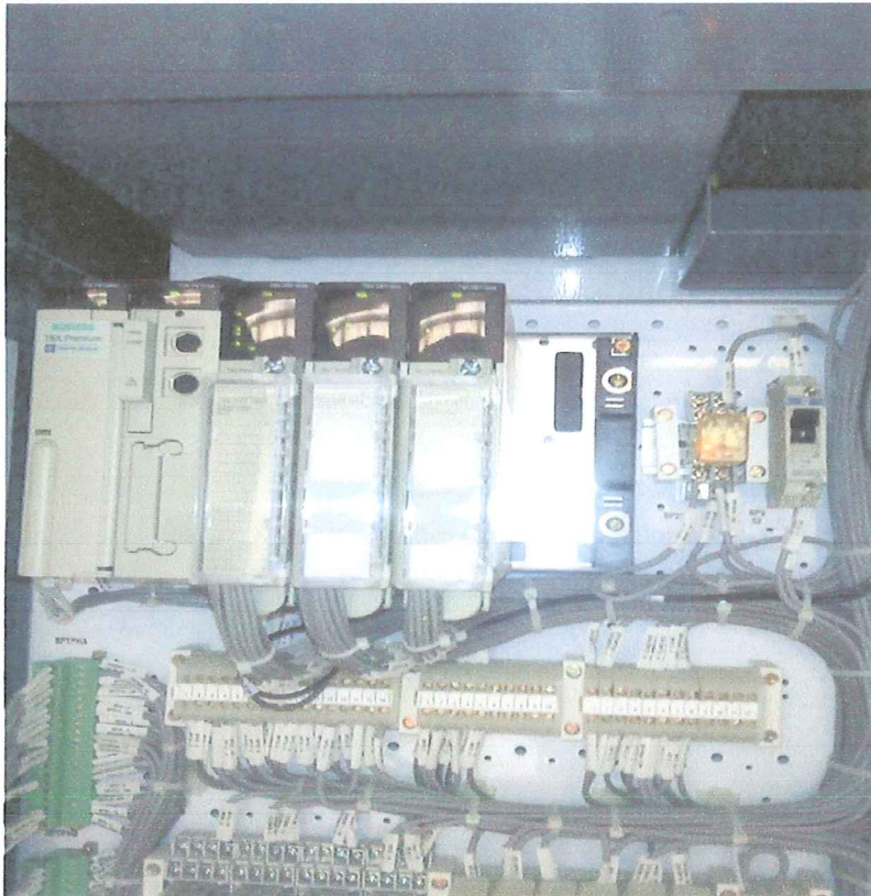
PLC for generator transfer switch.
