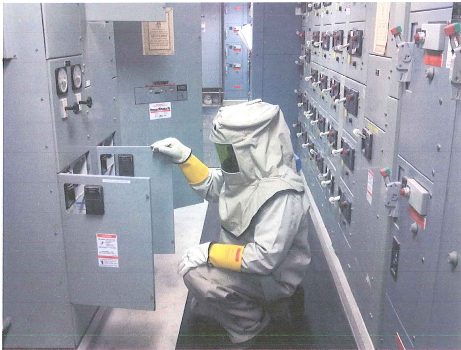
HVM technician in arc flash protective clothing to conduct Arc Flash Survey.
