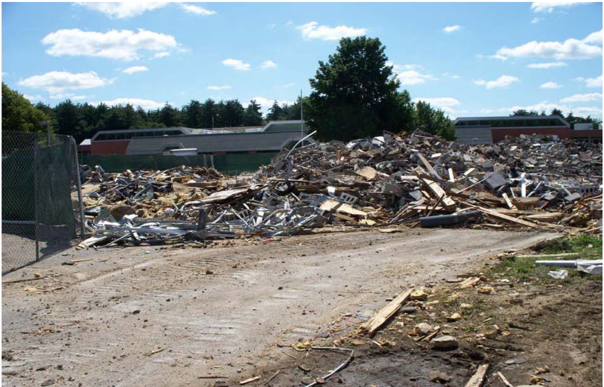
Demolition of Old Willard School nearly complete on Sept 1 (New School is in background)
