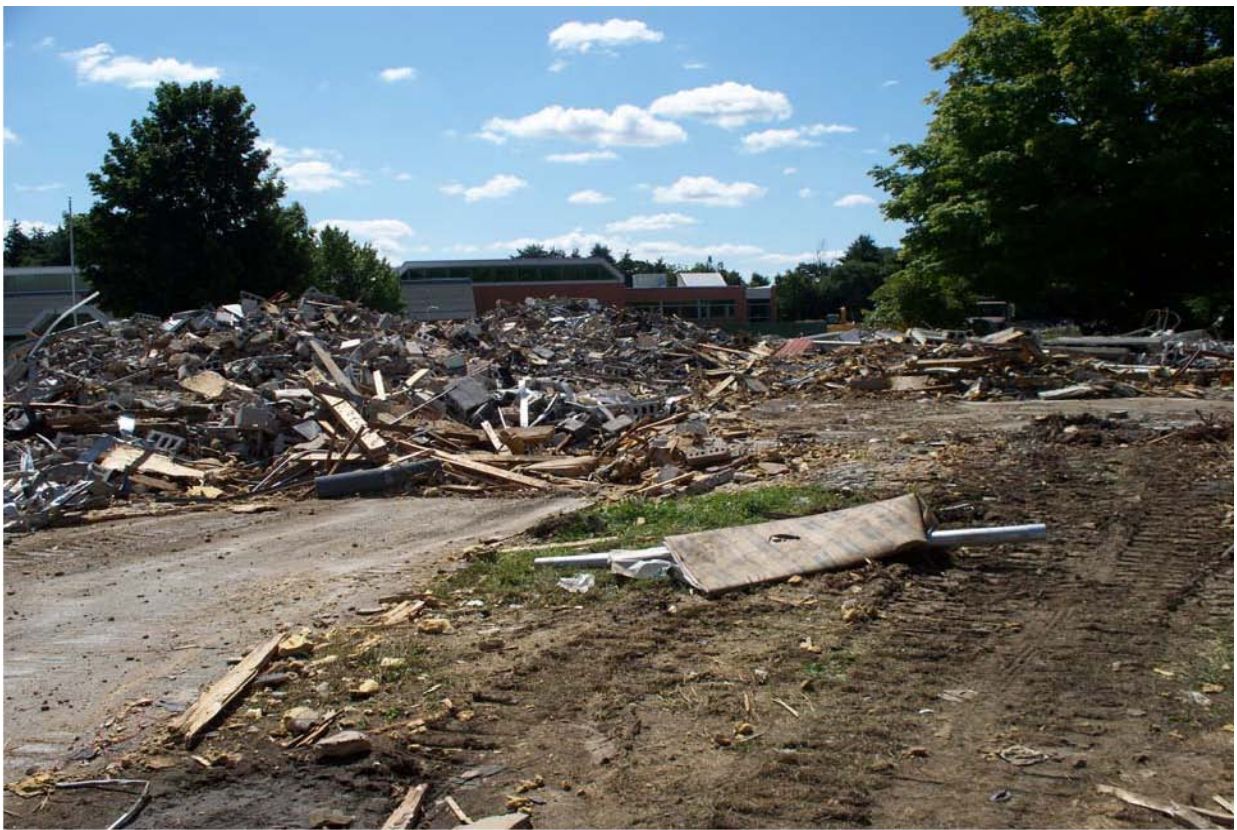
Much of the former Willard School Building will be sorted and recycled
