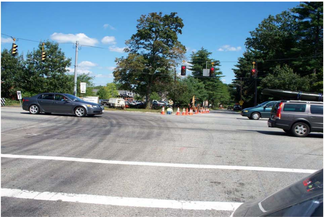
National Grid Crews Replacing gas main at intersection of Route 2 and ORNAC, addressing long-standing gas leak problems.
