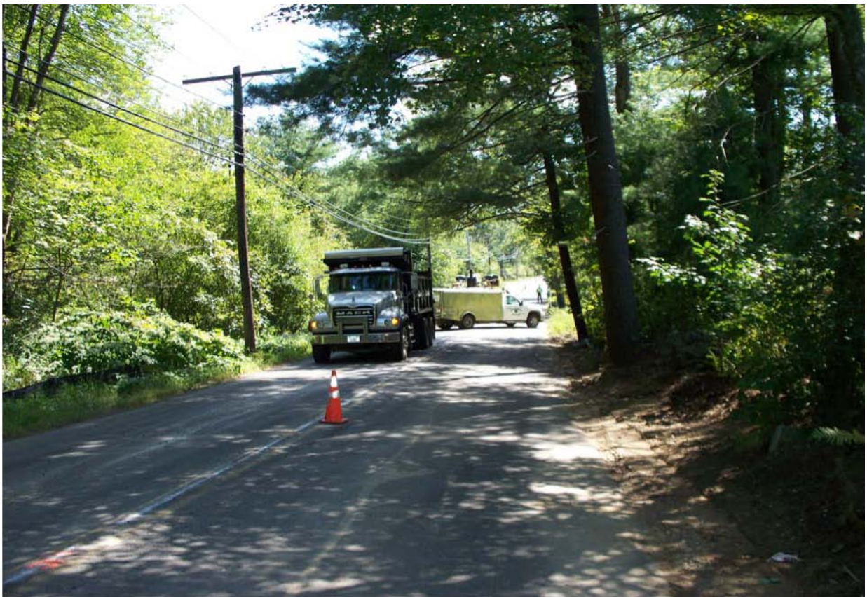
Top Course of Paving being installed on ORNAC (9/1/09) - following 2008 installation of water line connecting White Pond Well with new Deaconess Water Treatment Facility.
