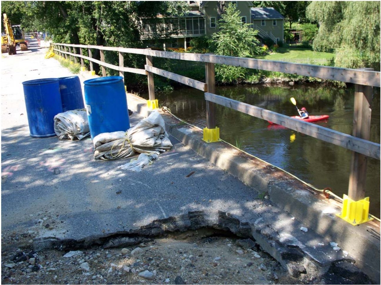
Work on Flint Bridge (Monument St) Suspended Pending further instructions from Mass Highway
