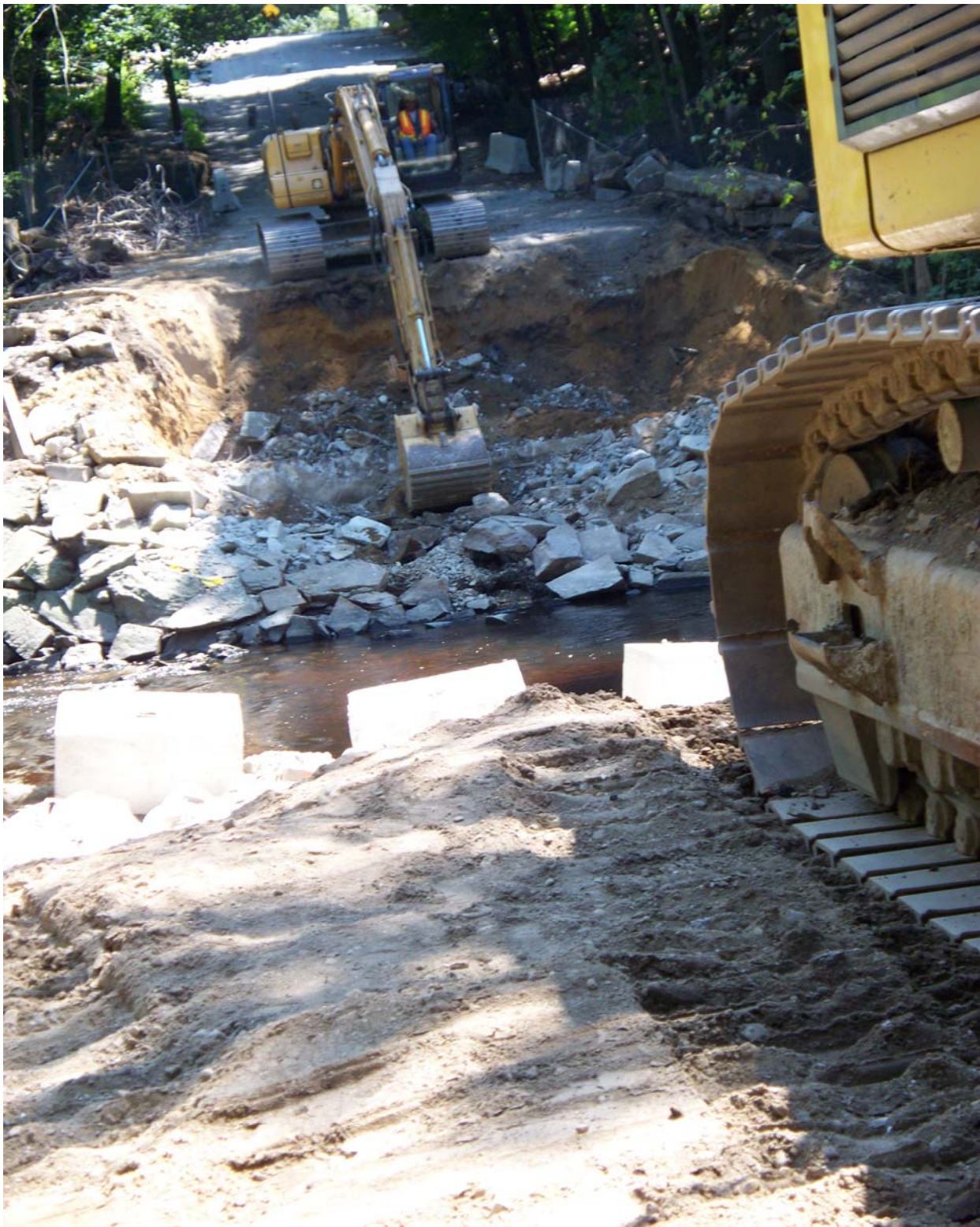
The Pine Bridge Has Been Demolished and Removed. The Upland Road approach is being prepared.
