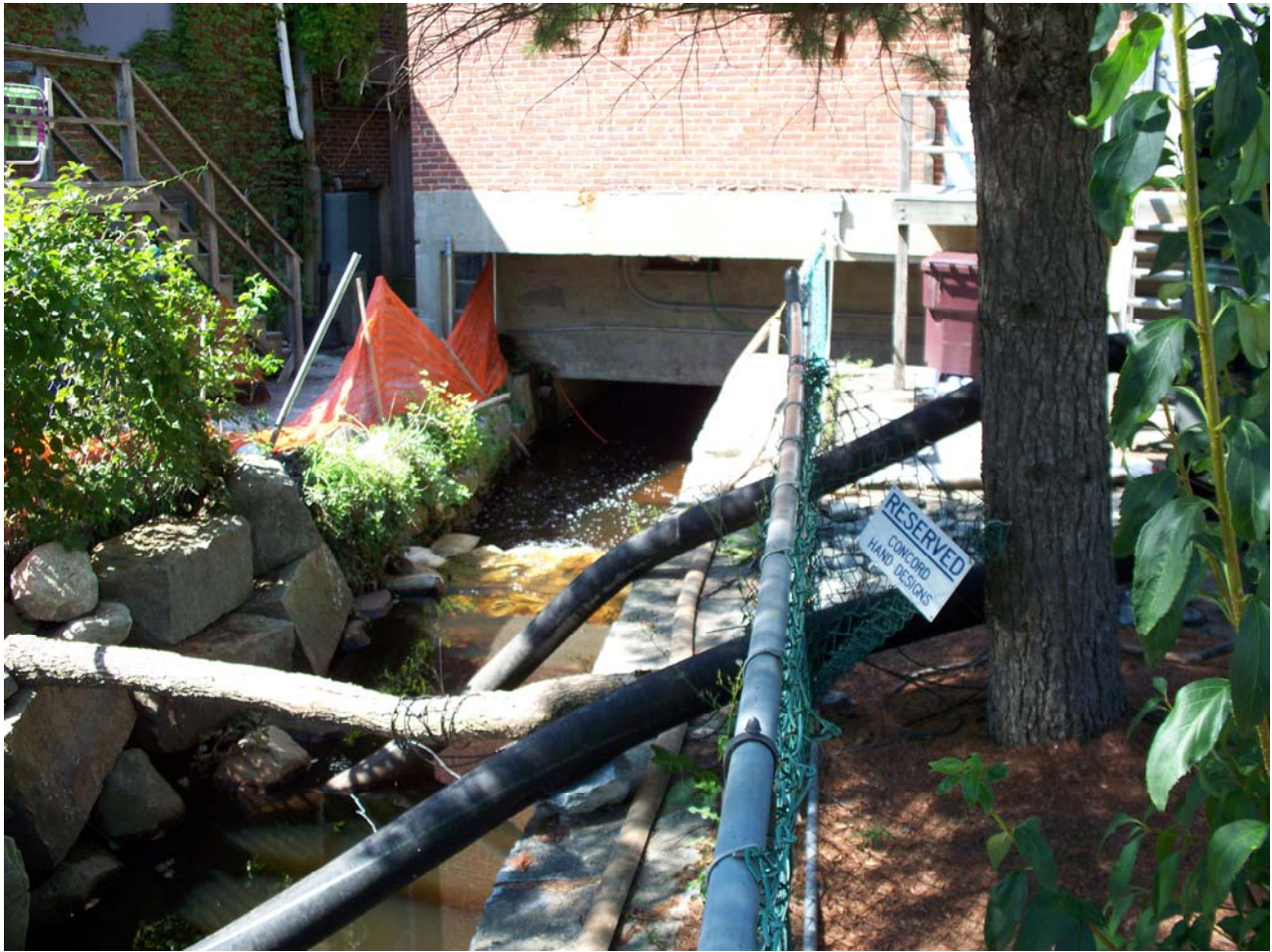
Work on Milldam Culvert under Main St Suspended due to high water levels
