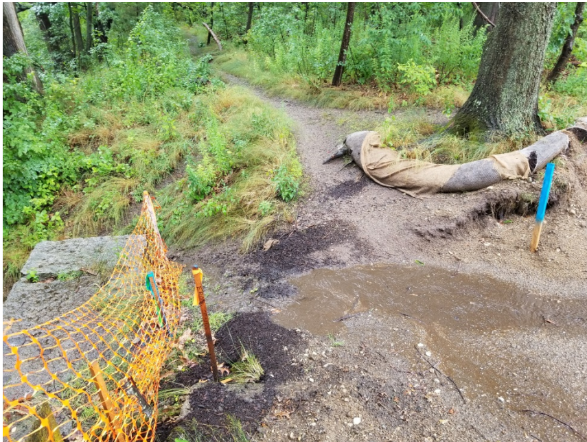
EROSION CONTROL IN NEED OF REPAIR.
