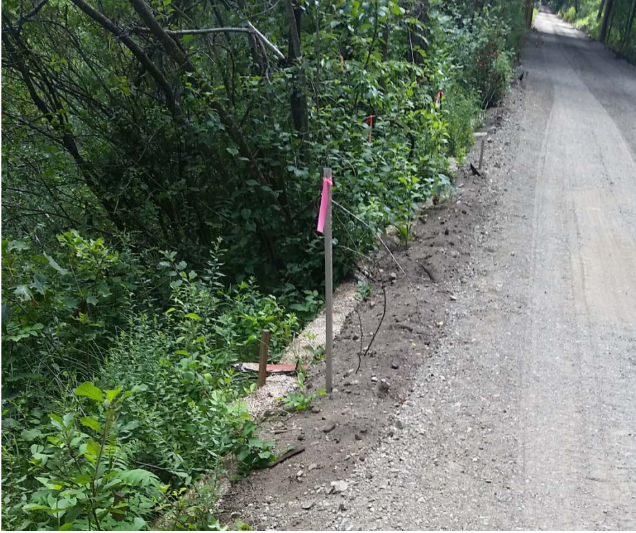
NEWLY SUBGRADED AREA, REQUIRING REPAIR OF EROSION CONTROL
