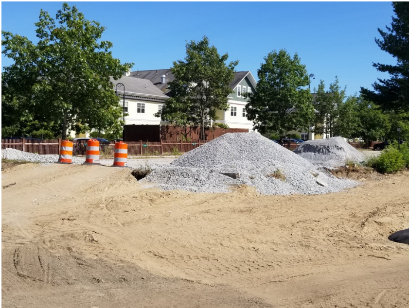
BUILDING MATERIALS STOCKPILES OUT OF REGULATED AREAS
