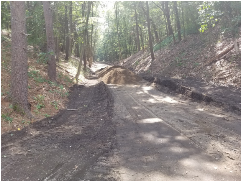
STOCKPILED SOIL OUTSIDE OF REGULATED AREA
