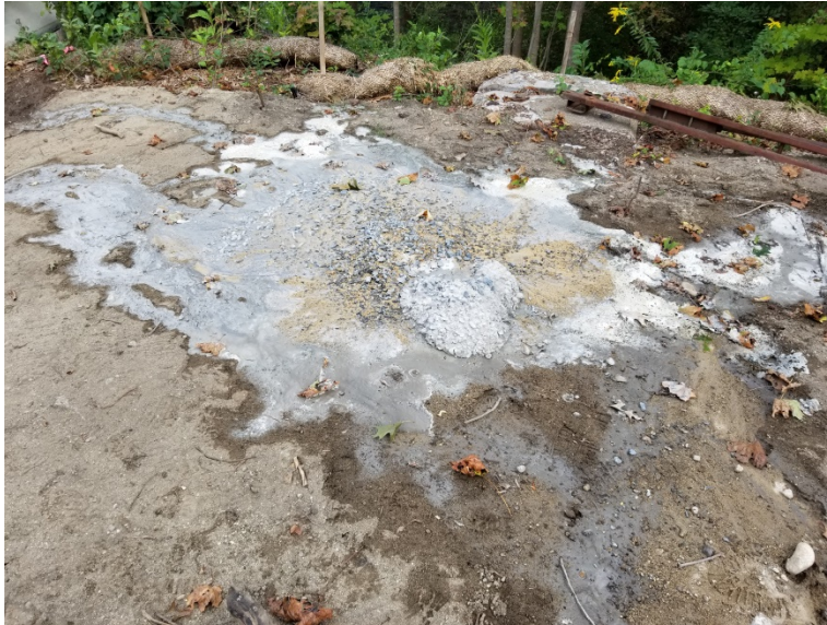
IMPROPER EXCESS CONCRETE WASHOUT
