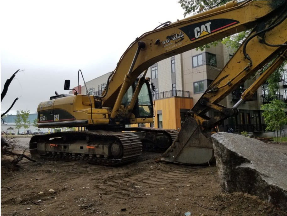
EQUIPMENT STORED WITHIN REGULATED AREA
