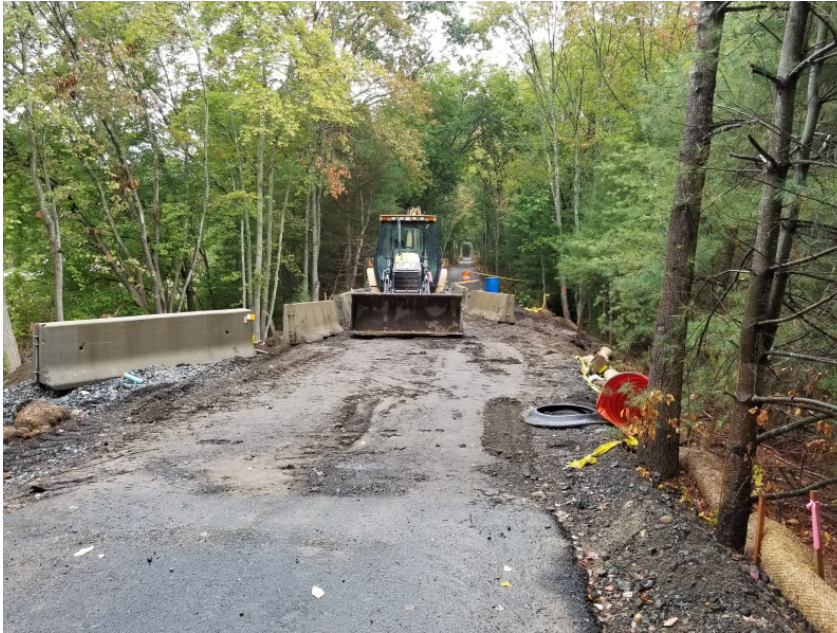
EQUIPMENT STORED WITHIN REGULATED AREA
