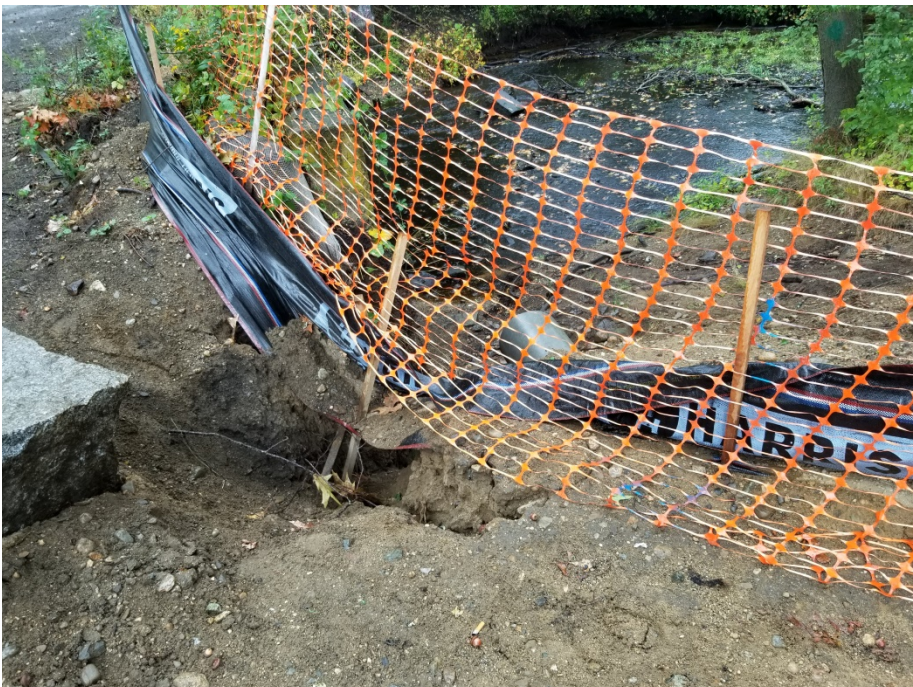
RECENT SEDIMENT WASHOUT
