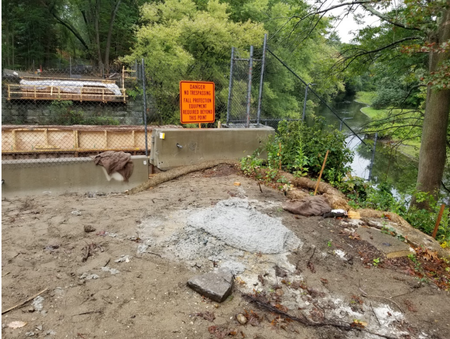
IMPROPER EXCESS CONCRETE DISPOSAL
