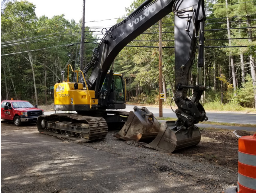
STORED EQUIPMENT OUTSIDE OF REGULATED AREA.
