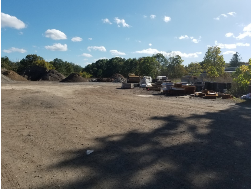
EROSION CONTROL AND CONSTRUCTION MATERIAL STORED OUTSIDE REGULATED AREA.
