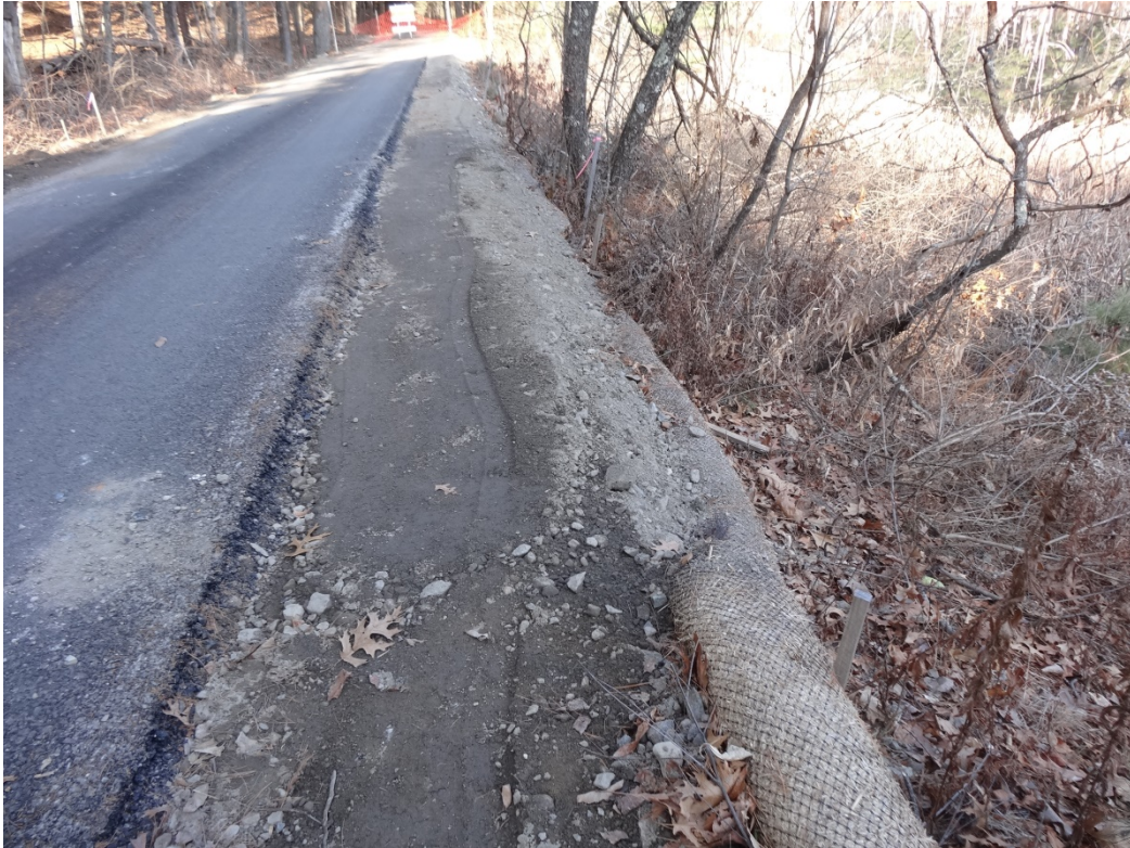
EROSION CONTROL WHICH NEEDS TO BE REPAIRED.
