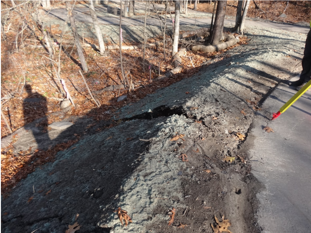
SEDIMENT WASHOUT LOCATED AT POWDER MILL ROAD HANDICAP RAMP.
