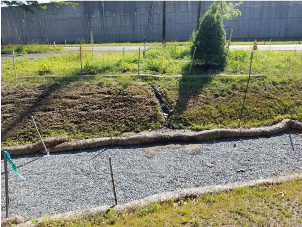
COMMONWEALTH AVE PARKING LOT DETENTION BASIN REPAIRED. NEEDS FURTHER MEASURES.
