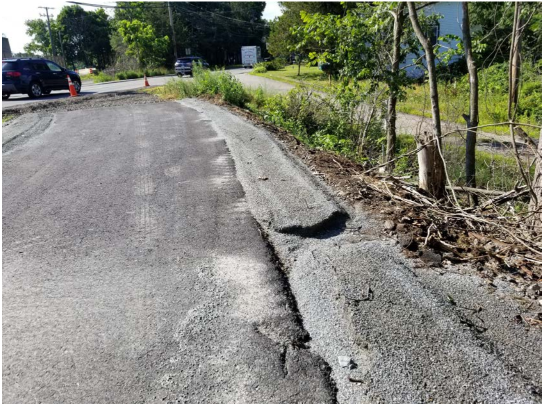
TYPICAL STONE DUST SHOULDER EROSION AFTER RAINFALL EVENT.
