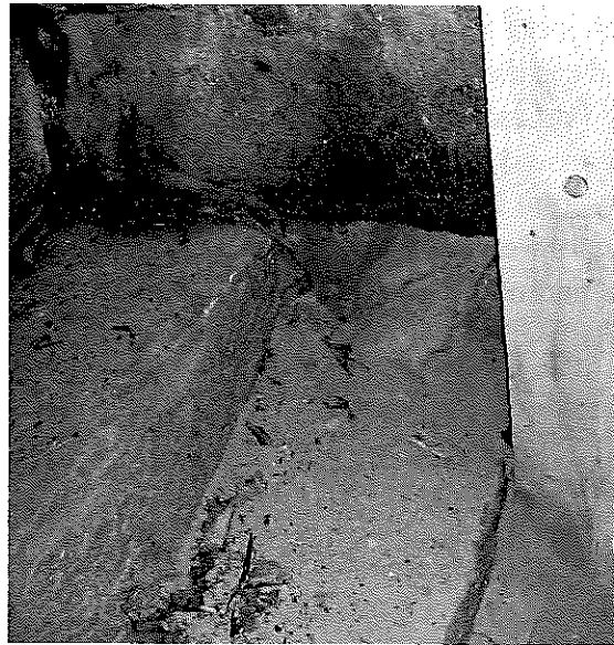
BULKHEAD STAIRS, OPEN JOINT
