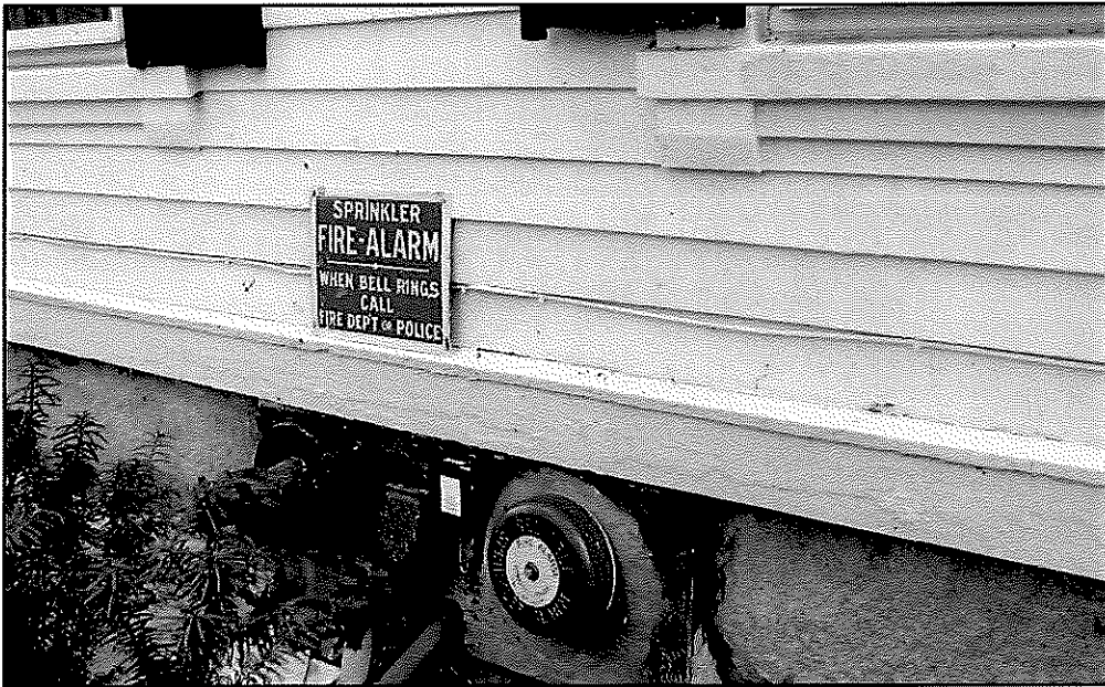
Figure 28: Water table trim board with sloped cap at bottom of clapboarded walls & above the stone foundation
