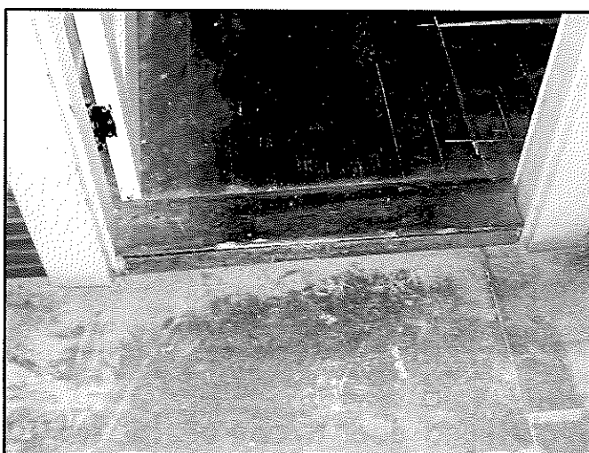
Figure 70: Attic flooring at doorway to northeast bedroom (oak flooring in bedroom; wide pine painted flooring in hallway)
