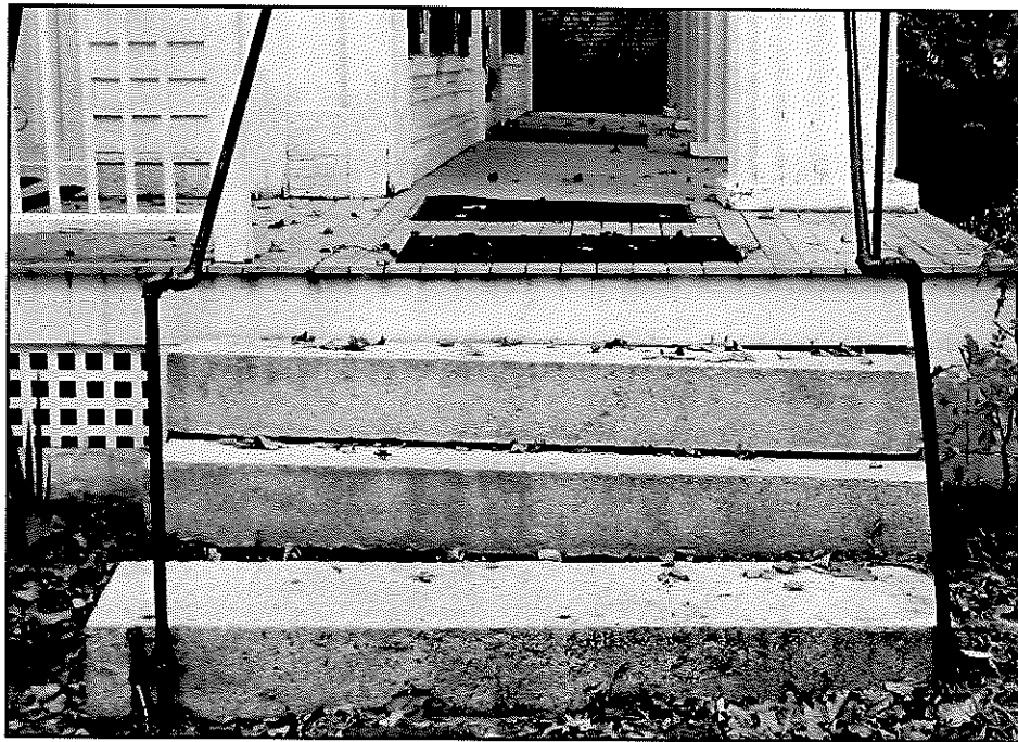
Figure 75: Connection of porch and front portico decks -- stone steps were moved and repositioned to accommodate the transition
