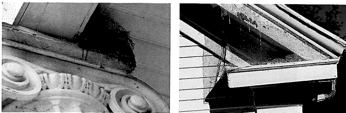
UNSIGHTLY WIRE MESH INSTALLED TO DETER BIRDS
