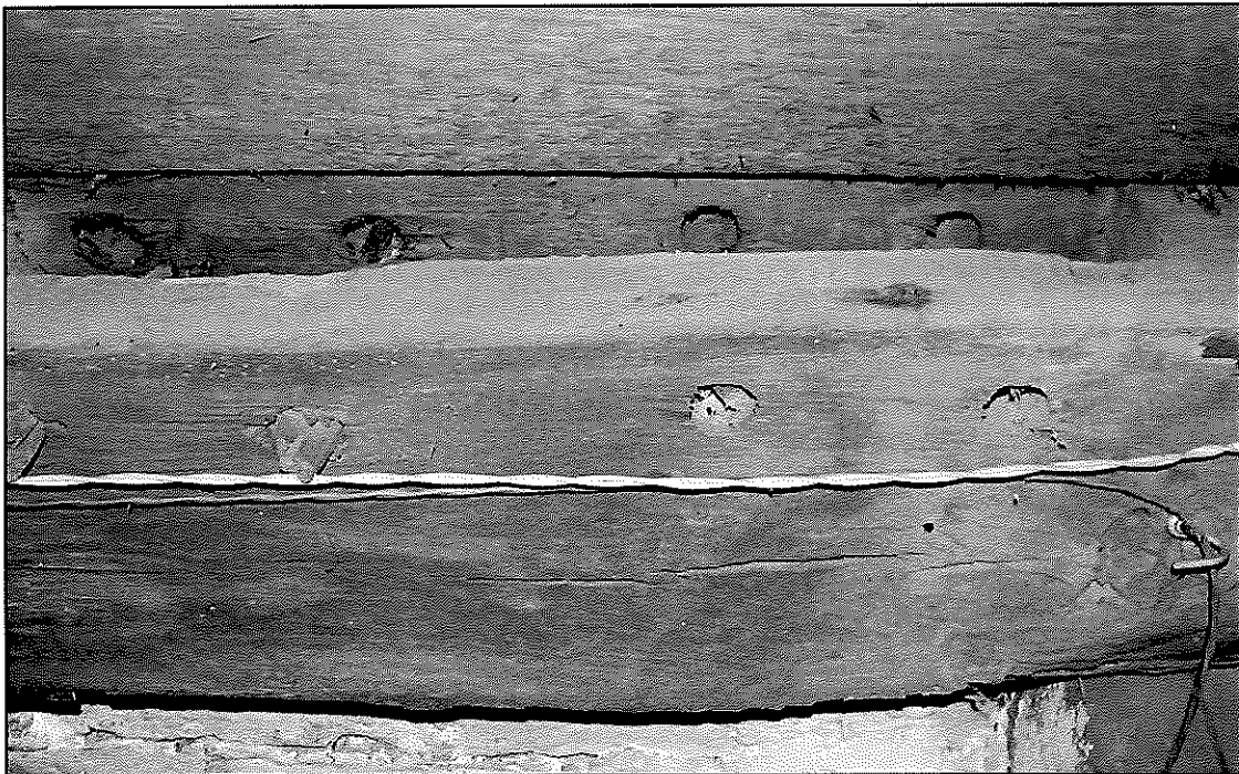
Figure 15: Re-used beam w/ double mortise and 4 pegs (next to west chimney foundation in cellar)
