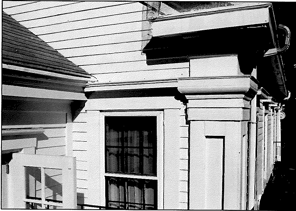
Figure 34: Intersection of ell roof east eaves with 2 nd floor window cap at main house south wall, southeast corner
