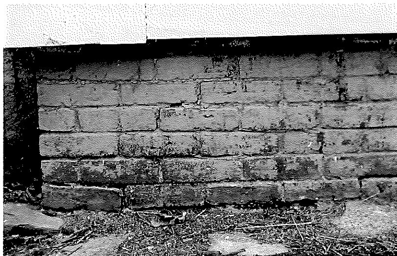
OPEN JOINTS AND MISALIGNED BRICK IN FOUNDATION
