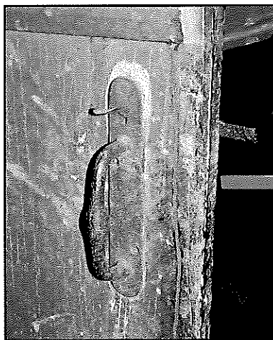
Figure 56: Front and back sides of door to room in NW corner of cellar (top), and original cast iron latch (bottom)
