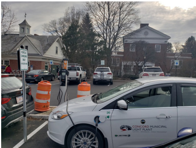
EV Charger - Keyes Rd Parking Lot
