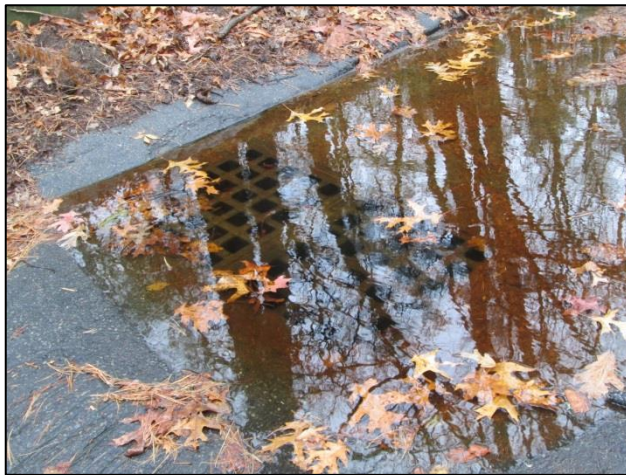
The catch basin at the White Pond public access boat launch quickly reached capacity, allowing untreated or minimally treated stormwater to flow directly down to the pond.
