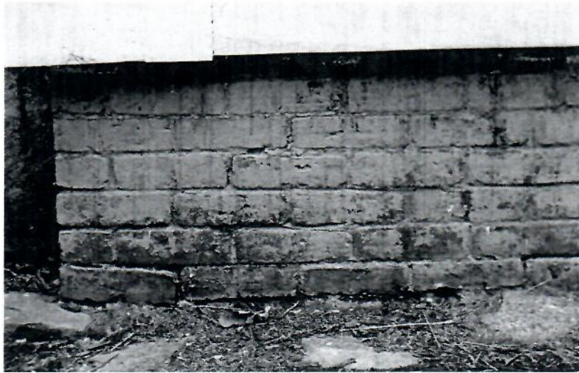
OPEN JOINTS AND MISALIGNED BRICK IN FOUNDATION
