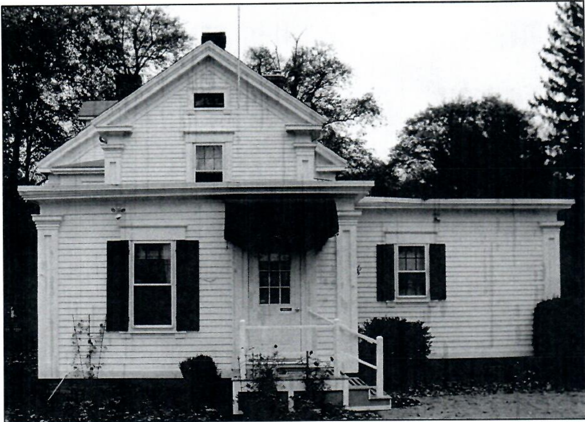
Figure 32: South wall of ell (with later one-story additions), showing original 2 nd floor window, and attic window in gable.
