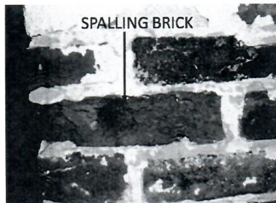
TYPICAL SPALLING BRICK IN BRICK PIERS AND CHIMNEY FOUNDATIONS
