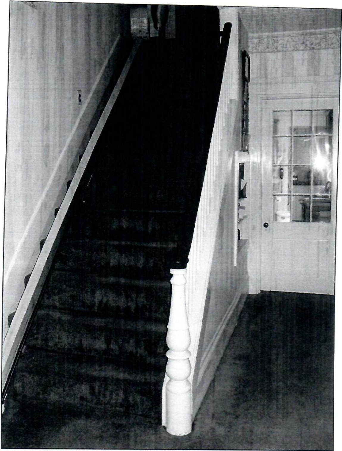
Figure 78: Rebuilt back stair to second floor, widened in 1977, newel post and railing salvaged from original stair (Original door w/ glass to kitchen seen at right, at end of back hallway)
