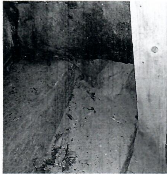
BULKHEAD STAIRS, OPEN JOINT
