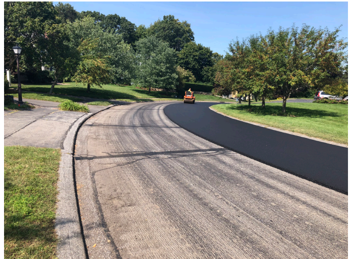
Partridge Lane Final Paving Design, Bidding and Construction of the 2021 Roadway Improvement Project
