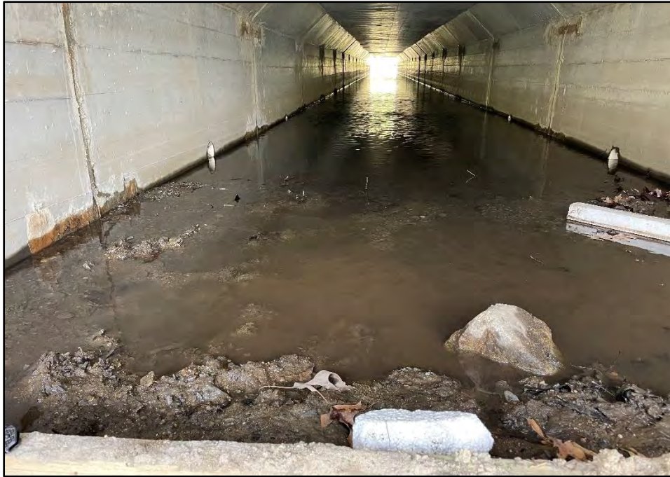
Photo 27. An additional view of the flooded tunnel after heavy rain, taken from the northern entrance.
