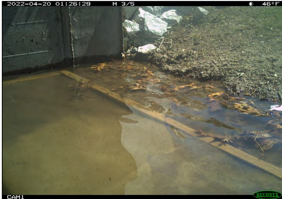
Photo 25. Frequent flooding of the tunnel as shown at the southern entrance above washed away track paths and likely prevented wildlife from successfully crossing.
