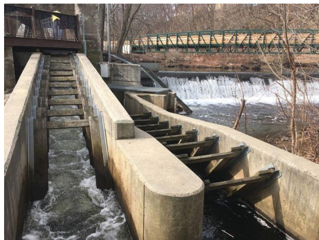
A typical Denil fish ladder.
