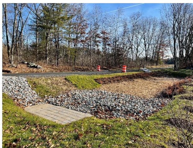
A small stormwater management system located along the Bruce Freeman Rail Trail at its crossing of Nashoba Brook north of Warner's Pond.
