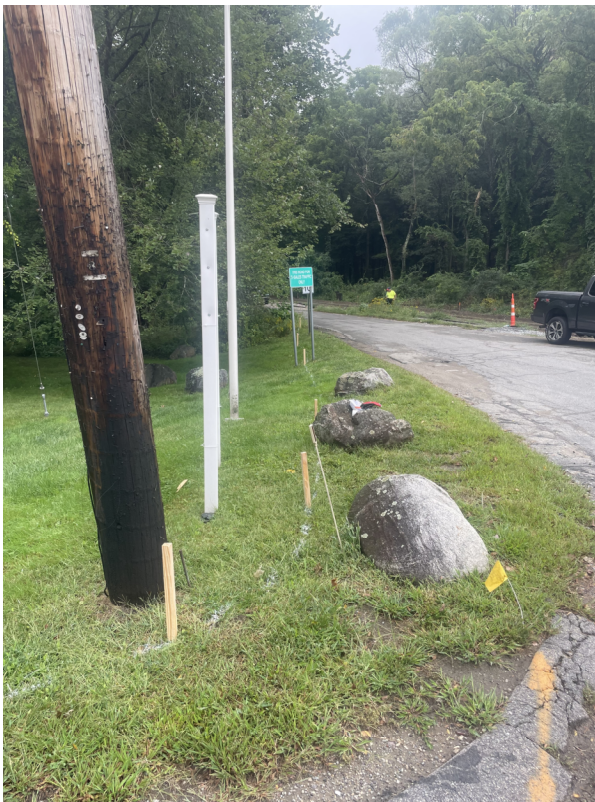
Photo 1: STA 175+50 looking North. Grade stakes placed at Ti Sales Driveway for new opening.
