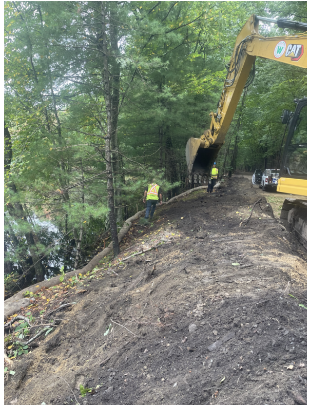
Photo 10. STA 332+00 looking North in between the wetland pond area and western limit of proposed trail. Side slope leading to pond appears to be in stable condition even after major rain events.
