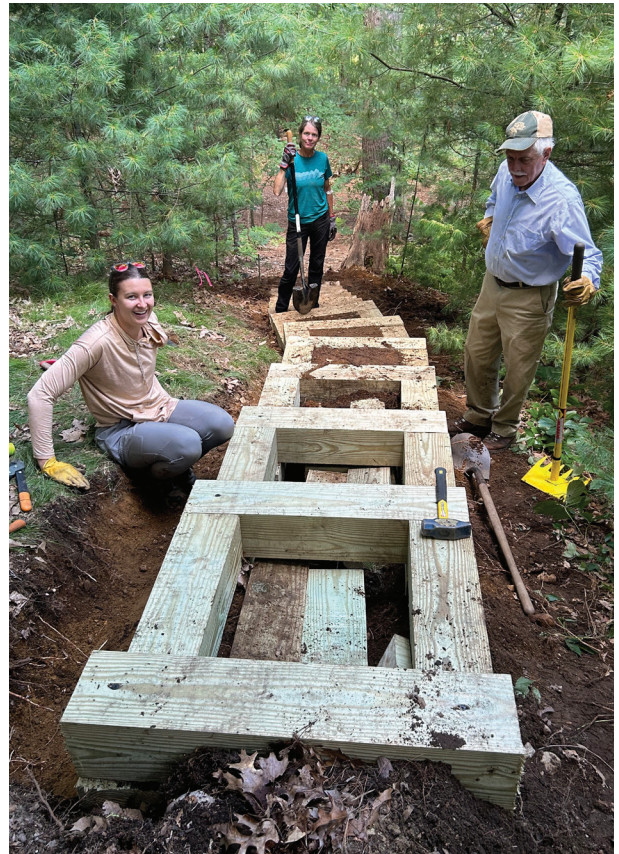
CLCT staff and volunteers built steps along the trail from Independence Rd. into Gowing's Swamp over the summer.
