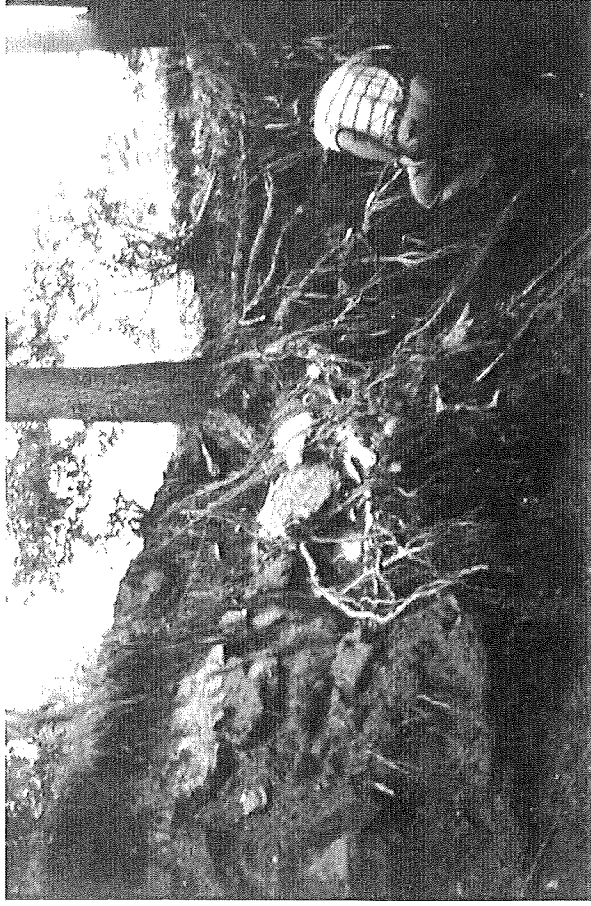
Tree root induced scouring on crest and downstream face of Coffey dam in Kansas
