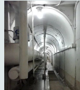
ISU steam tunnels
