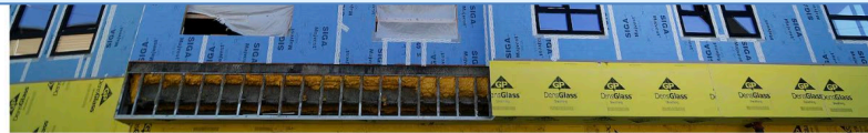
An affordable housing project under construction at 52 New Street in Cambridge. JOHN TLUMACKI/GLOBE STAFF
