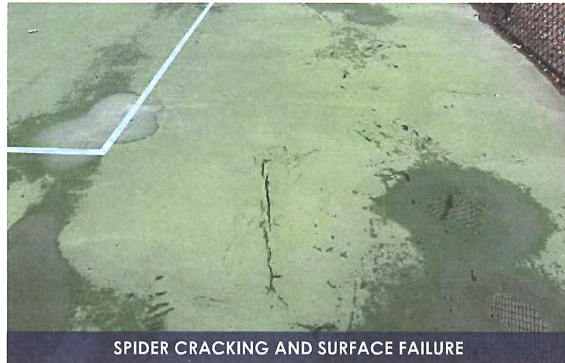
SPIDER CRACKING AND SURFACE FAILURE
