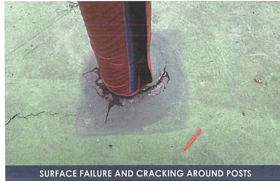
SURFACE FAILURE AND CRACKING AROUND POSTS
