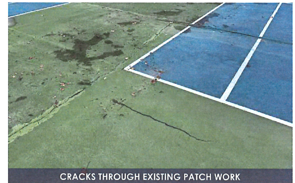
CRACKS THROUGH EXISTING PATCH WORK
