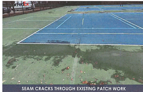
SEAM CRACKS THROUGH EXISTING PATCH WORK
