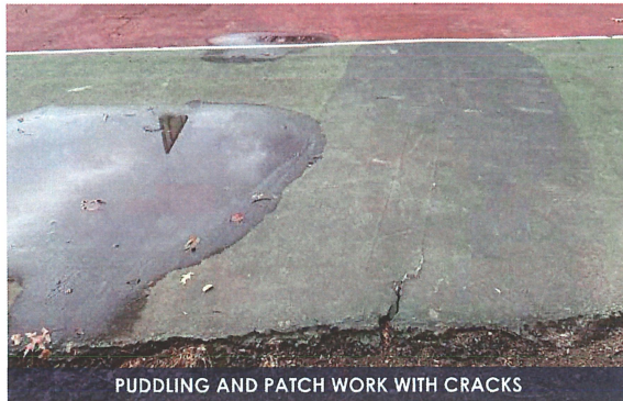
PUDDLING AND PATCH WORK WITH CRACKS
