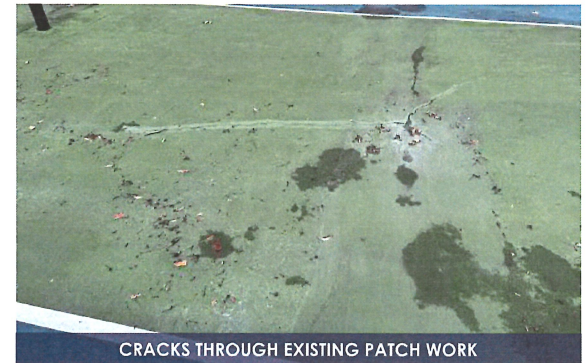
CRACKS THROUGH EXISTING PATCH WORK
