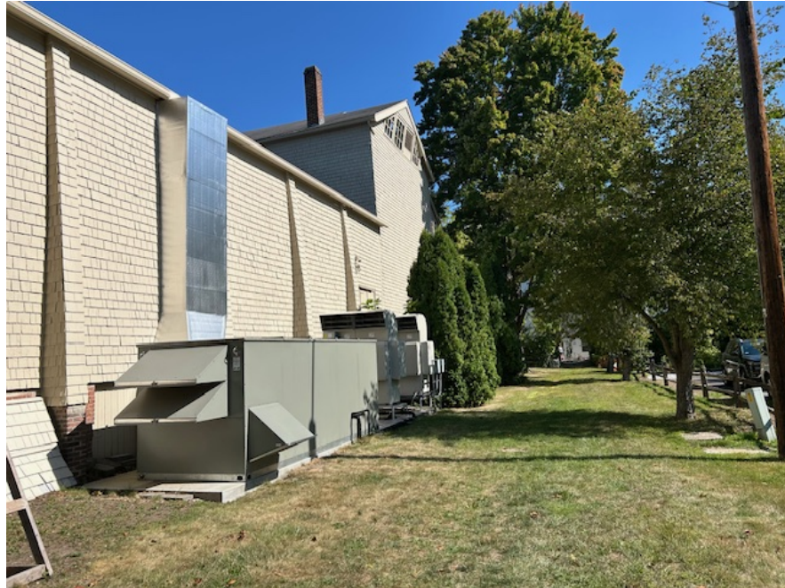
Exterior air handlers and pumps
