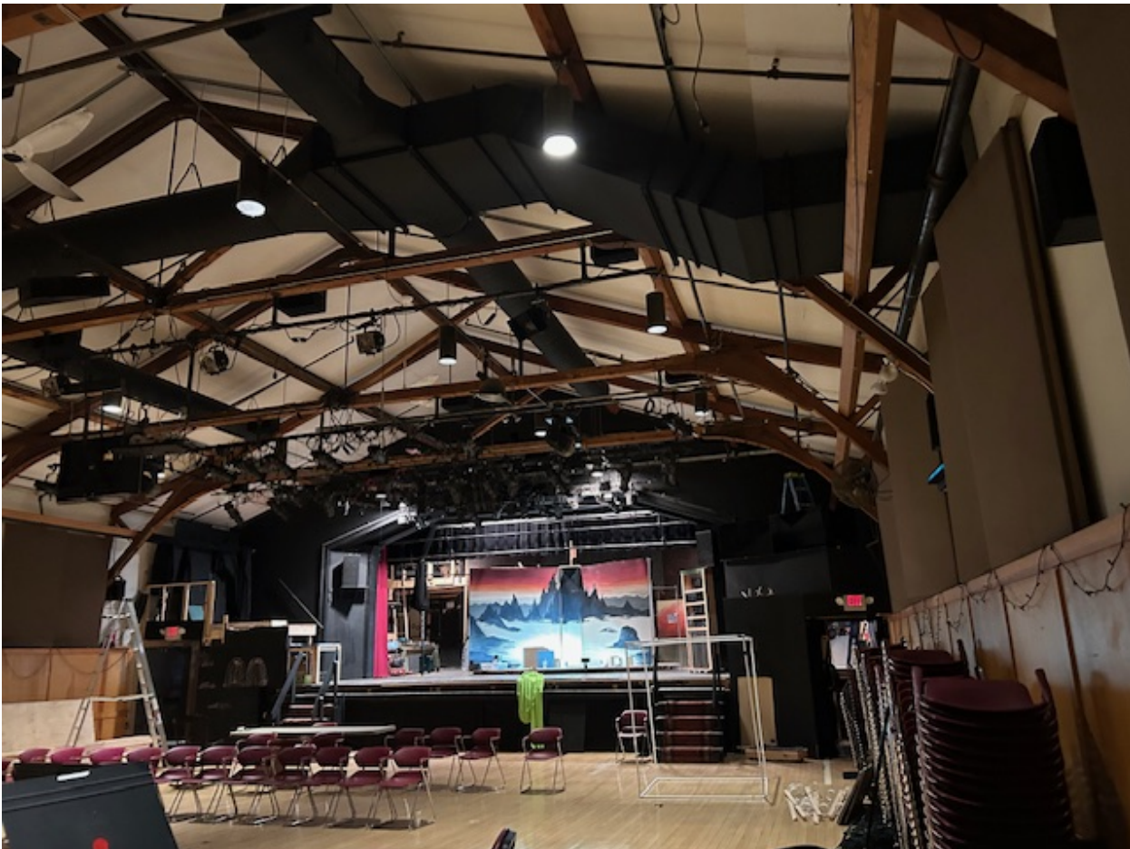
Ductwork in the hall
