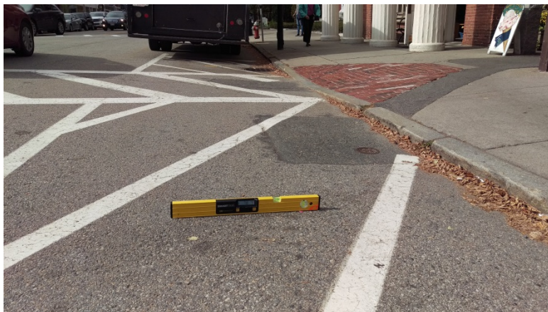
Figure 13: Excessive roadway cross-slopes within Main Street (7.1%)
