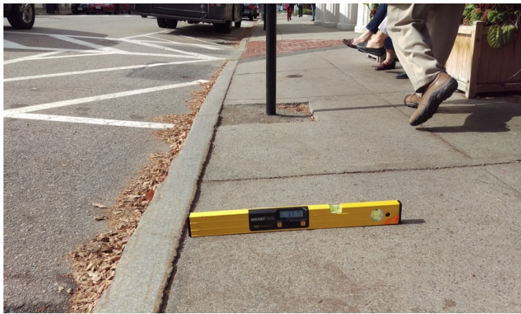
Figure 12: Excessive sidewalk cross-slopes within Main Street (3.7%)
