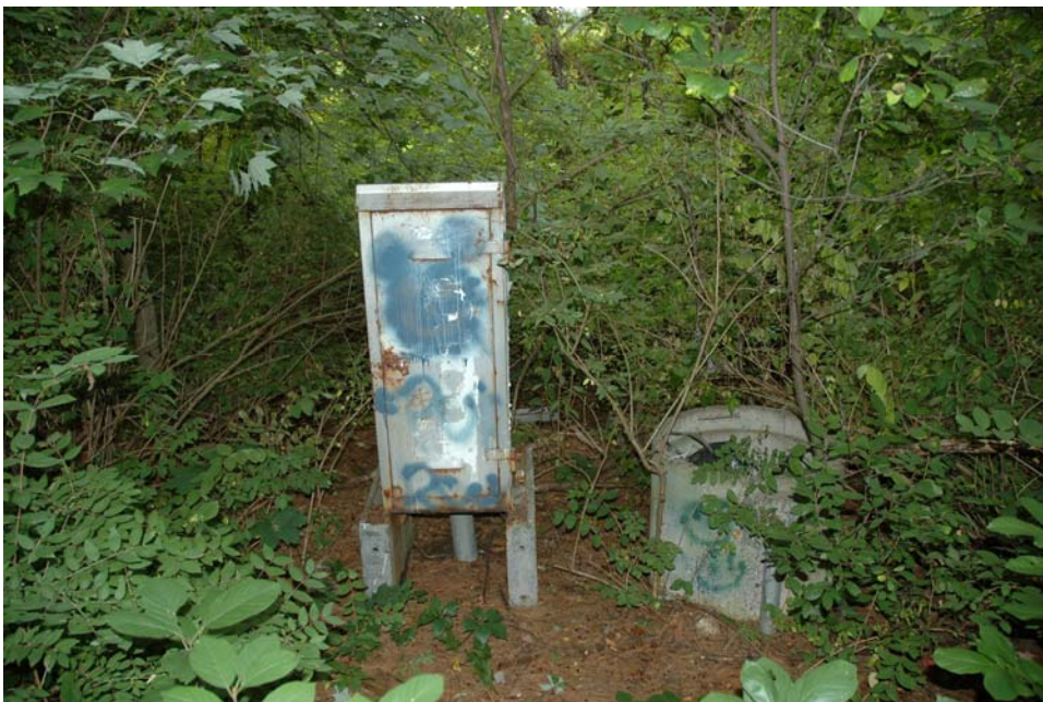
Photo 34. Resource 35, Relay box, looking west.
