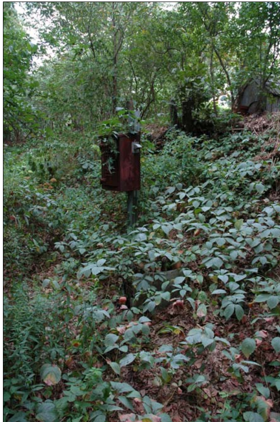
Photo 31. Resource 31, Relay box, looking northeast.
