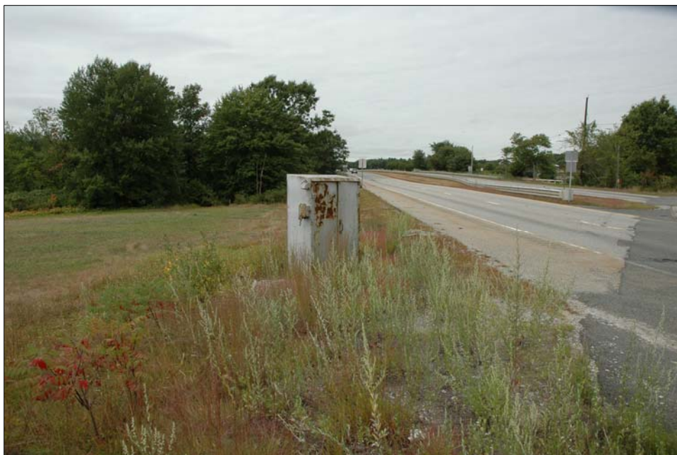
Photo 2. Resource 2, Relay cabinet, looking northwest.
